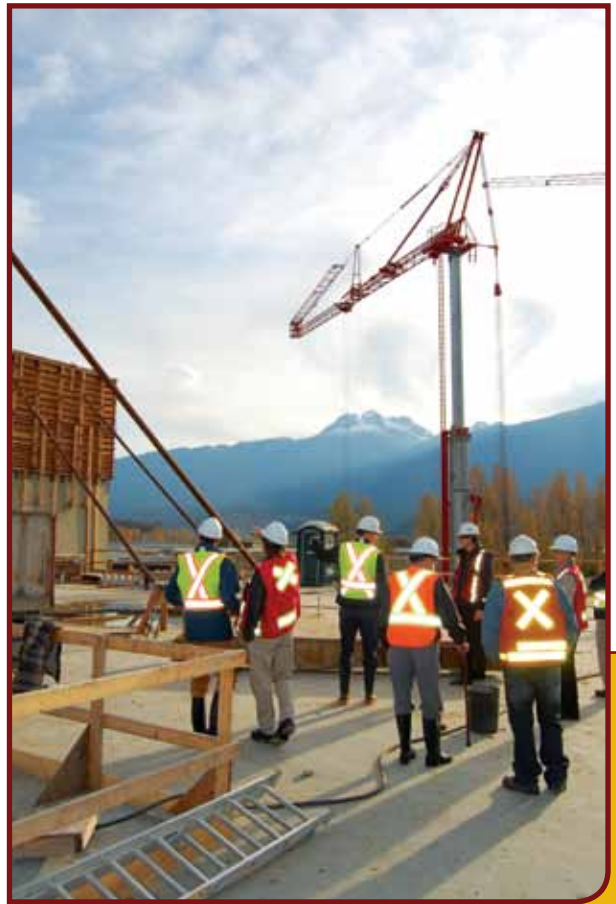
New school construction site, Photo: Courtesy of David Rooney, The Revelstoke Current
